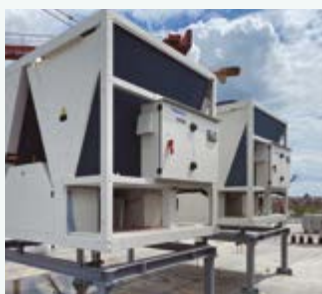
CÉDRUS LIGET, a complex facility including apartments, penthouses and showrooms etc. Hungary. ECOi-W - ECOi - PACi
