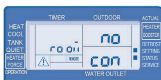
1. Connection of a room thermostat (YES/NO, Standard: NO)
